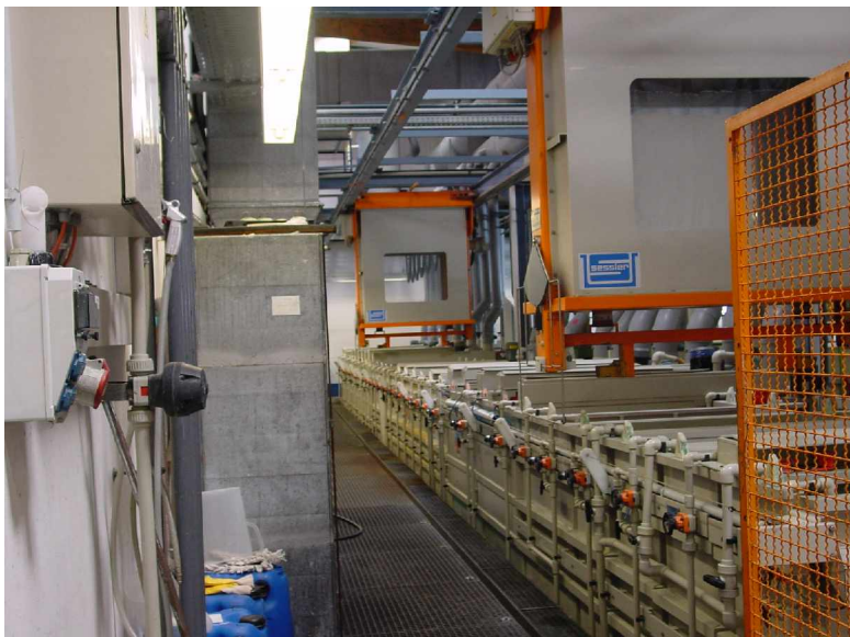
Figure 9: Automatic galvanisation plant (Schaal)
